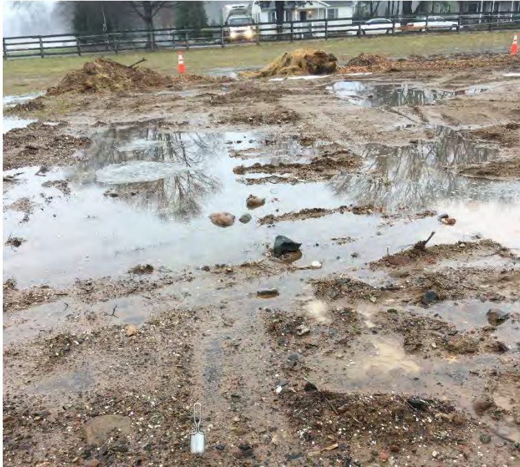
Photo 4. Ponding near site 3.
